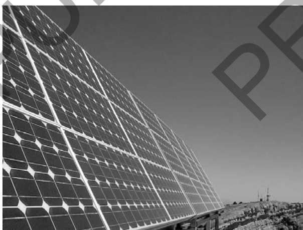
Figure 7. Solar Panels – Spain
