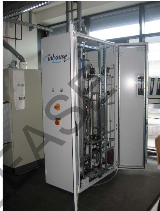
Figure 2. 5kW fuel cell facility for mobile tests.
