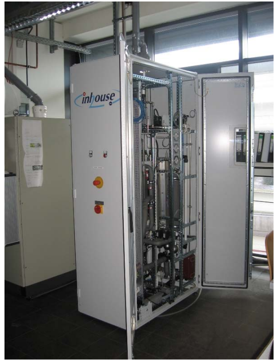
Figure 2. 5kW fuel cell facility for mobile tests.
