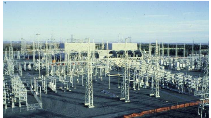
Fig 4. Nicolet convert station in transmission line Québec - New England
